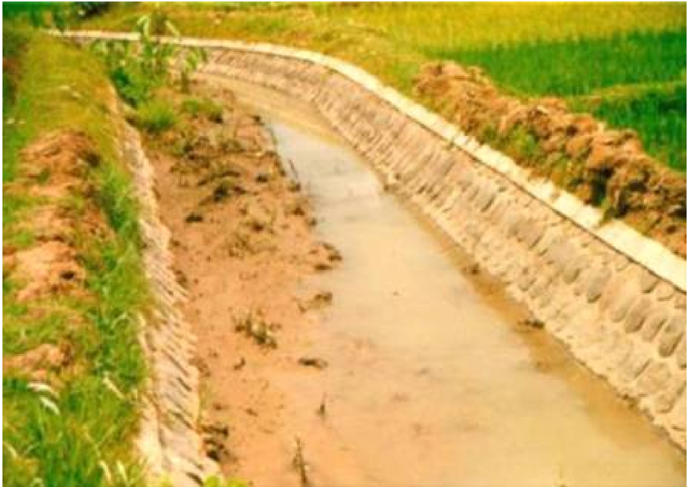
Siltation in Canal
