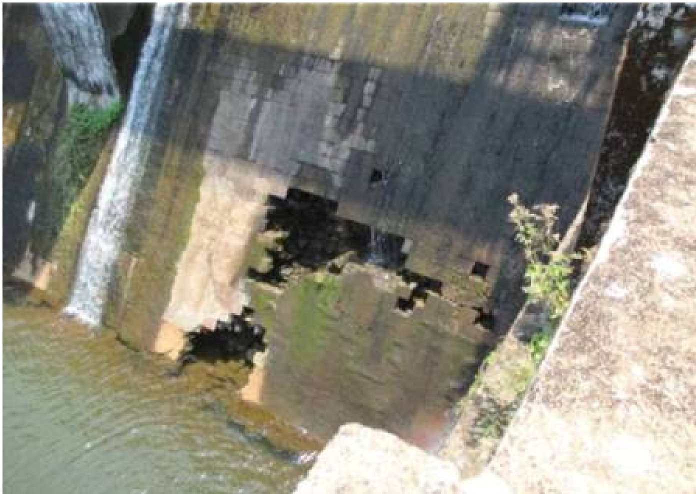
Poor Maintenance of Structure
