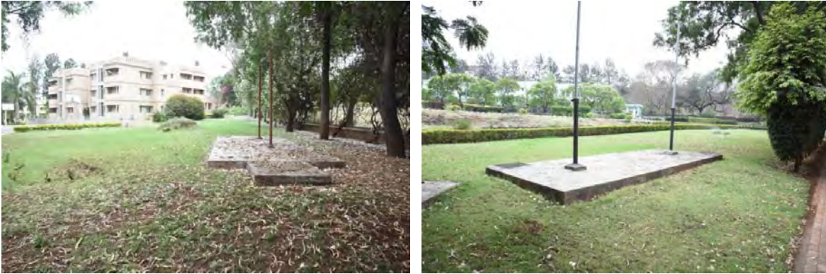
Figure 10. Safe Disposal of Waste Water using Septic Tanks within NWA Campus
