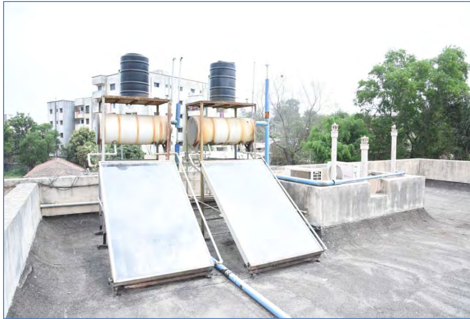
Figure 33. Rooftop Solar Panels
