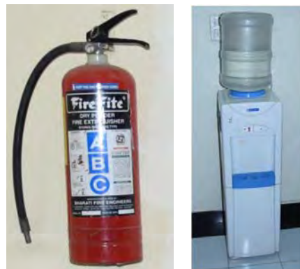
Figure 29. Fire Fighting Equipments and Water Cooler
