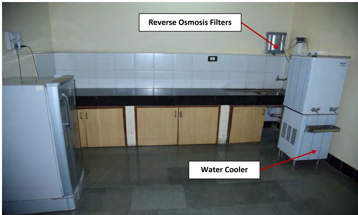
Figure 19. Potable/RO treated Water and cooler at NWA Campus
